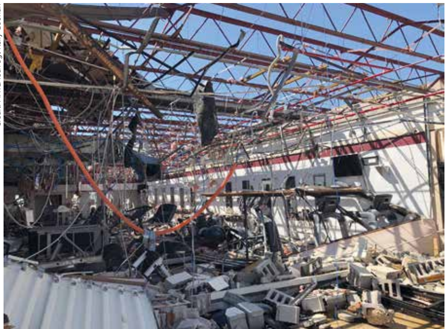
A Tyndall AFB building in the aftermath of Hurricane Michael. Much of the base suffered extensive damage to infrastructure.
