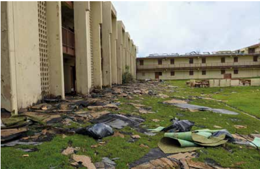
The aftermath of Typhoon Mawar landing in Guam. The total damage to military facilities on the island was estimated at USD 10 billion.
