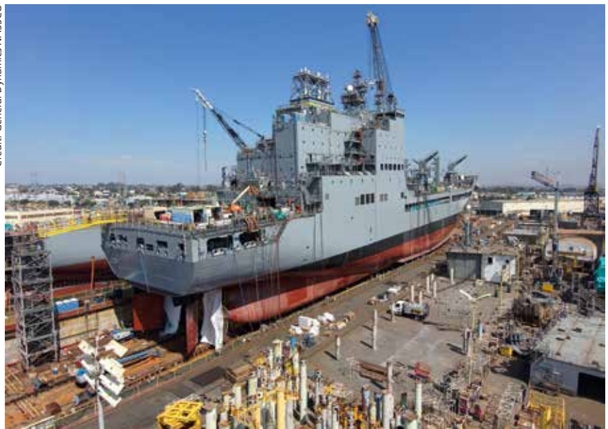
The third John Lewis class fleet replenishment oiler, Earl Warren (T-AO-207), pictured during construction by General Dynamics NASSCO. The photo shows the twin skeg arrangement, with two shaft-lines and twin rudders, that is increasingly common in modern replenishment vessel design.
